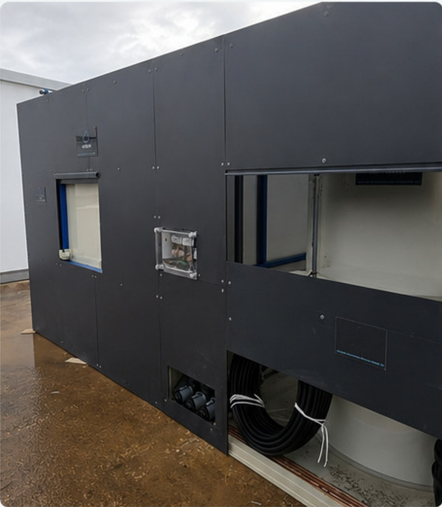
Service connections at the unit
