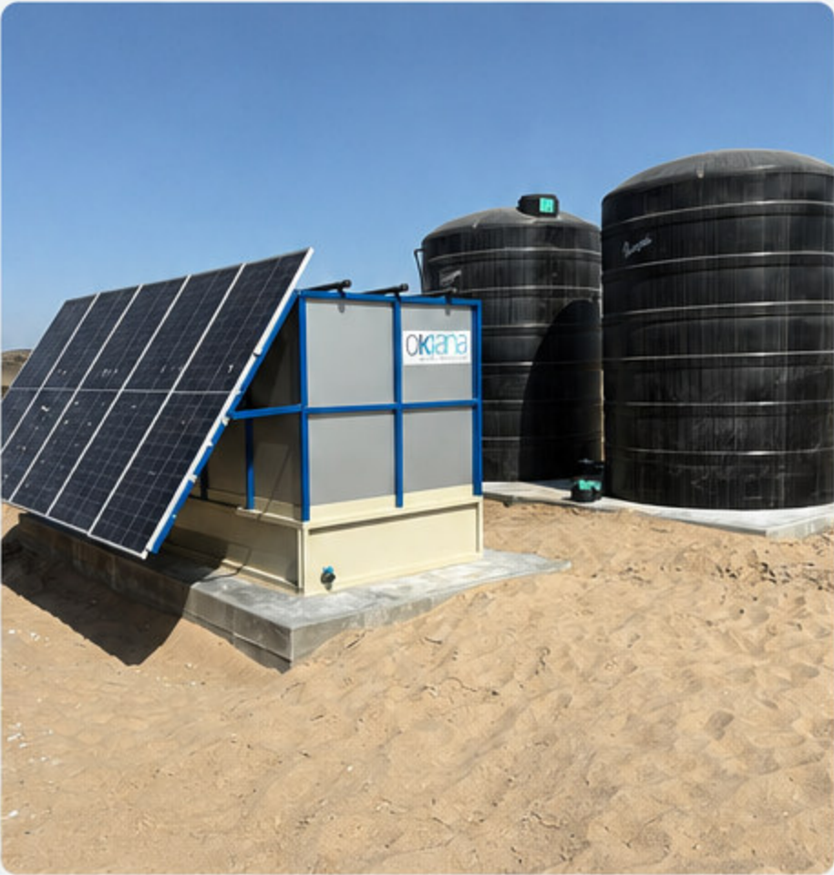
Solar array and storage tanks
